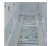
Air Shower Room
