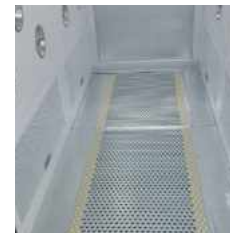
Air Shower Room
